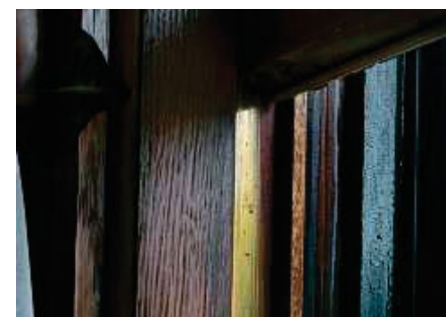
Metal glide strips were added to the window runners to allow smoother operation.
